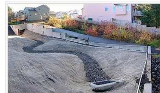
Two bioswales for a housing development. The foreground one is under construction while the background one is established.
