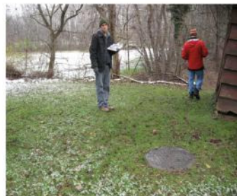
Manhole leading to the underground pipe that will be diverted to treatment areas.
