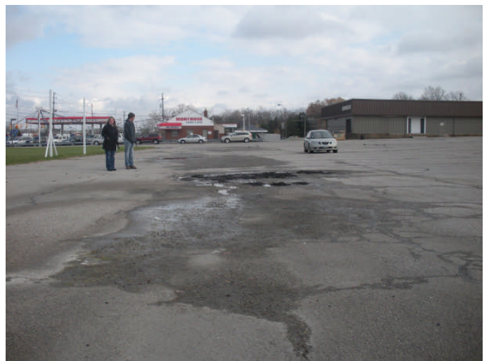
View of parking lot erosion
