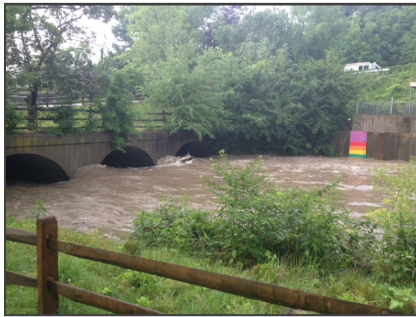
Flood waters entering triple culverts in Zoo
