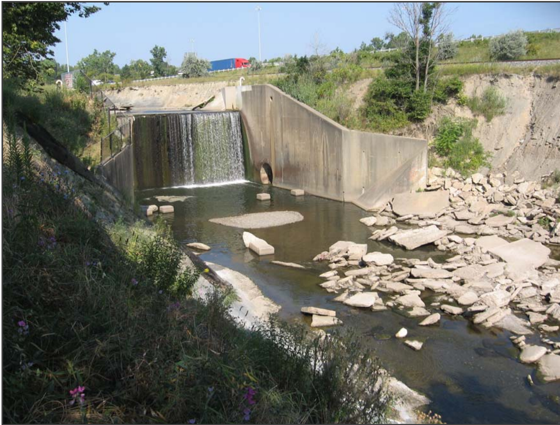
Big Creek Drop Structure or Spillway, Brookside Reservation, August 2013, showing CSX rail line and I-71 beyond.
