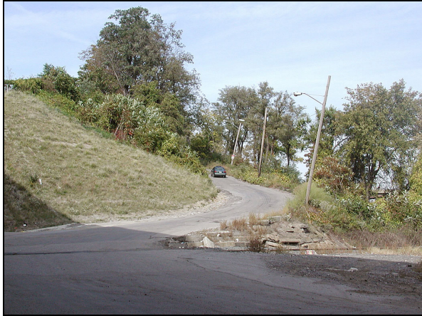
West 14 th Street is in poor condition for vehicular traffic
