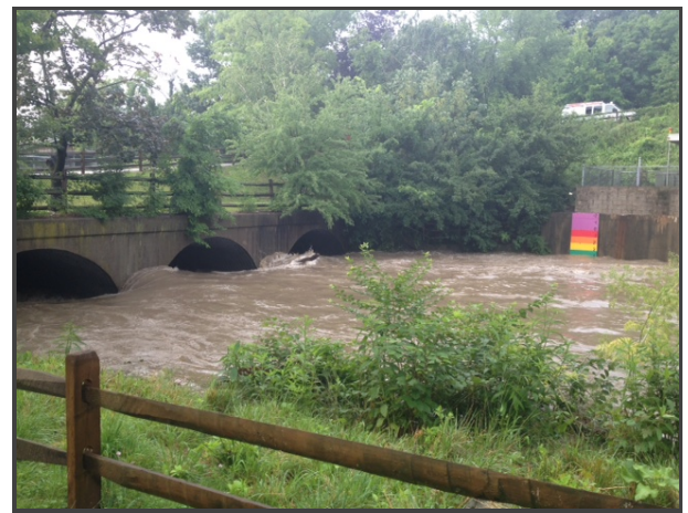
Flood waters entering triple culverts in Zoo
