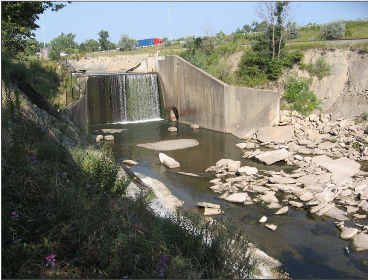
Big Creek Drop Structure, Brookside Reservation, August 2013, showing CSX rail line and I-71 beyond.
