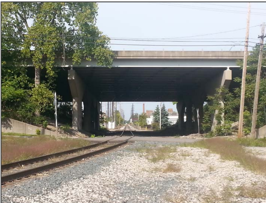
Denison Access ramp over NS railway, looking west. Tradex Parkway is to the left.
